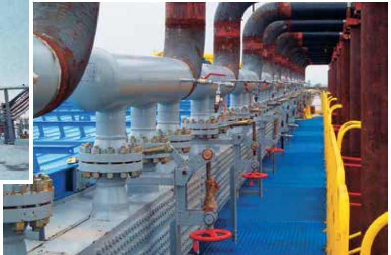
Right: Compressor building at the Lukoil Nahodkaskaya site in Western Siberia
