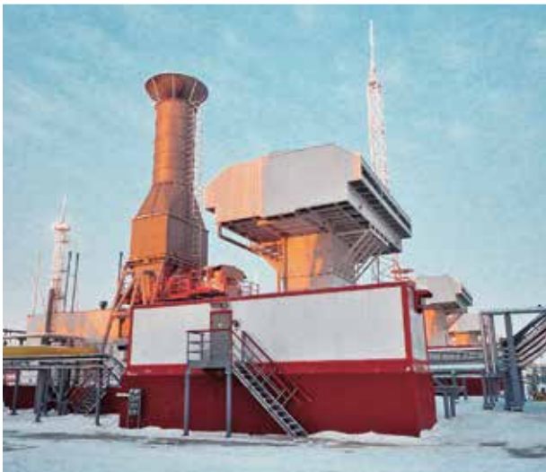
Top of facing page: Natural gas compressor at the Lukoil Nahodkaskaya site in Western Siberia
